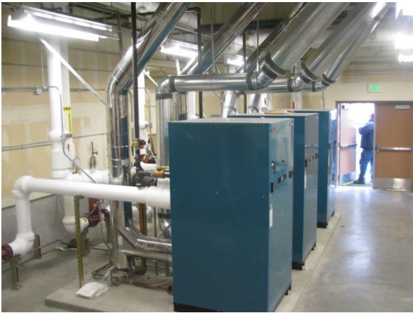
Bonney Lake HS: Modern HVAC Systems
